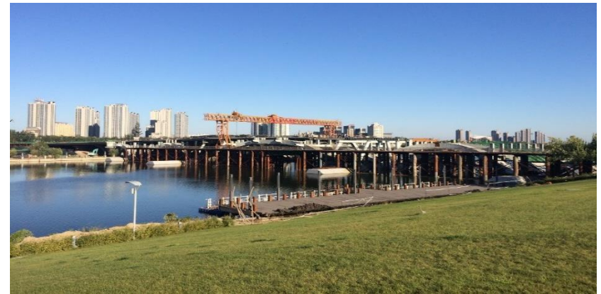
Construction of Bei Guan Avenue Yun He Bridge, connecting the development to a largely-residential precinct across the Grand Canal, is progressing well.
