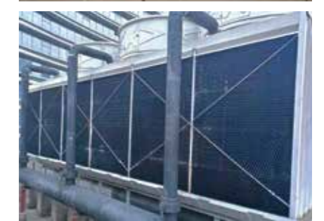
Before and after the replacement of roof cooling tower fillers at Perennial Qingyang Mall
